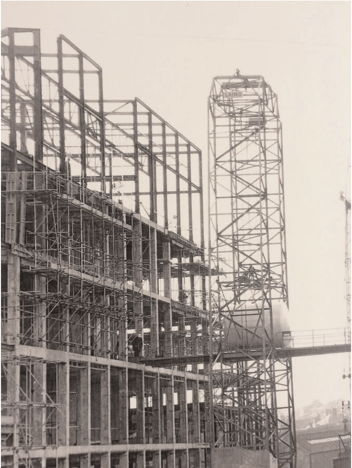
Figure 4. A special lift used to install horizontal tanks without the use of costly cranes. Courtesy of Martin Smith.
