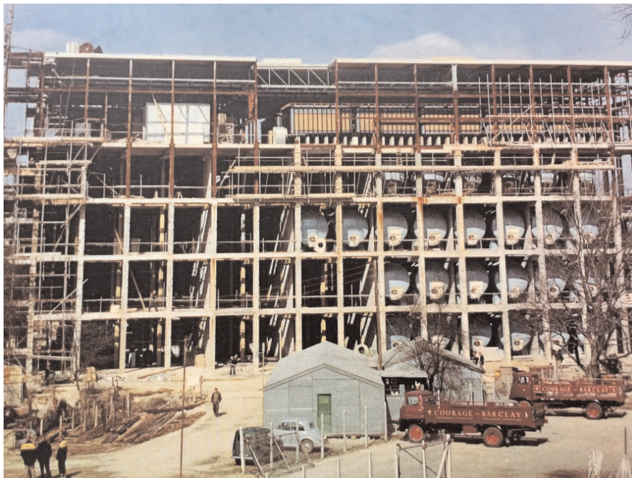
Figure 3. Main front of the brewery showing tanks before cladding. Courtesy of Martin Smith.
